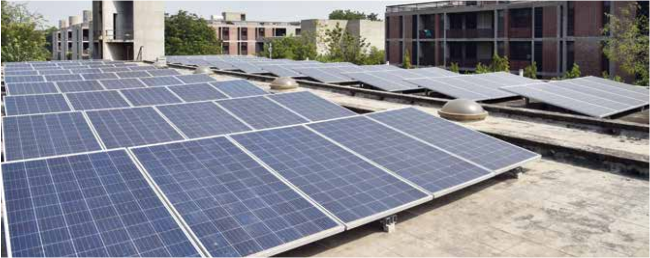
First Solar Power Plant at IIMA
