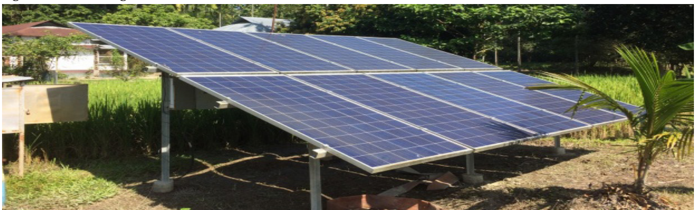
Figure 1: A Solar Irrigation Panel Installed in a Farm.
